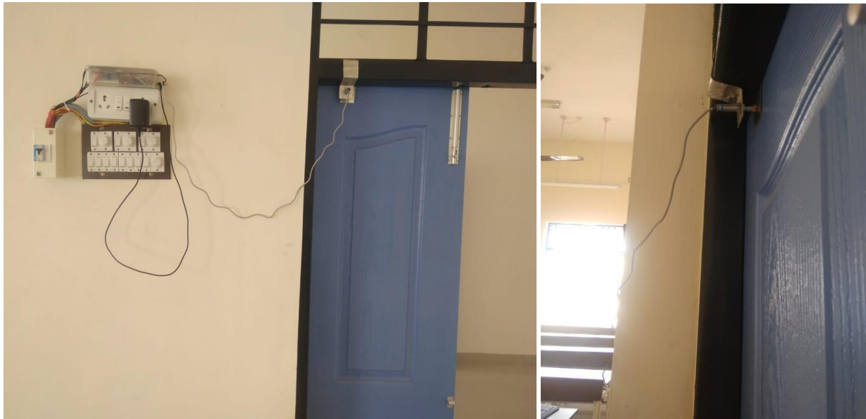
Fig: Proximity Metal Sensor Fixed in Door of Smart Class Room
